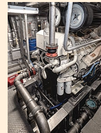
Two Cummins QSK38-M main engines, above, deliver a combined 2,600 horsepower through Twin Disc gears.
